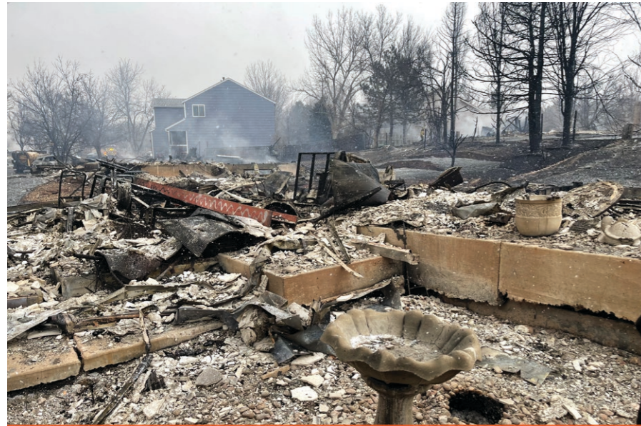
Wildland urban interface fires can quickly escalate due to the proximity to flammable vegetation
